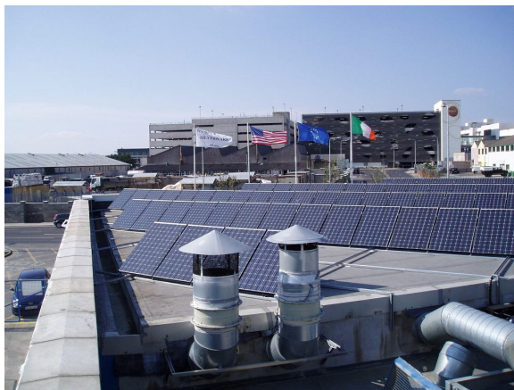
12.5 kWp system at Newbridge Silverware, commissioned by Coolpower in April 2007, part of 30 kWp in total at the site.
